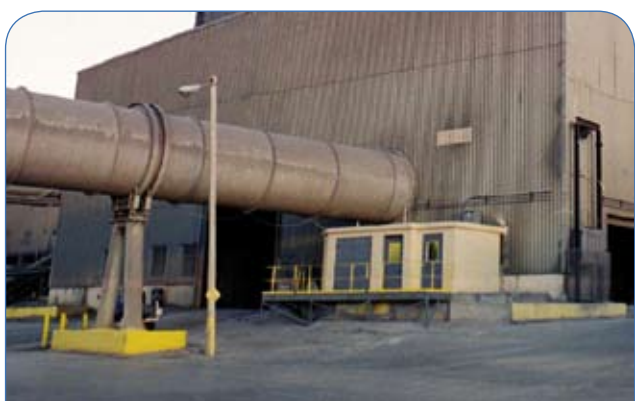
Figure 4. COSMA room installed under the product conveyor exiting the finish mill building at Ash Grove Cement, USA.
